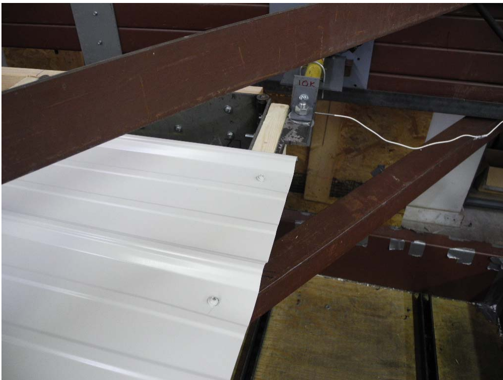
PHOTO 6 View of fastener tilting and panel slotting at the fastener near the loaded corner in Test #2. (DSCN1021)
