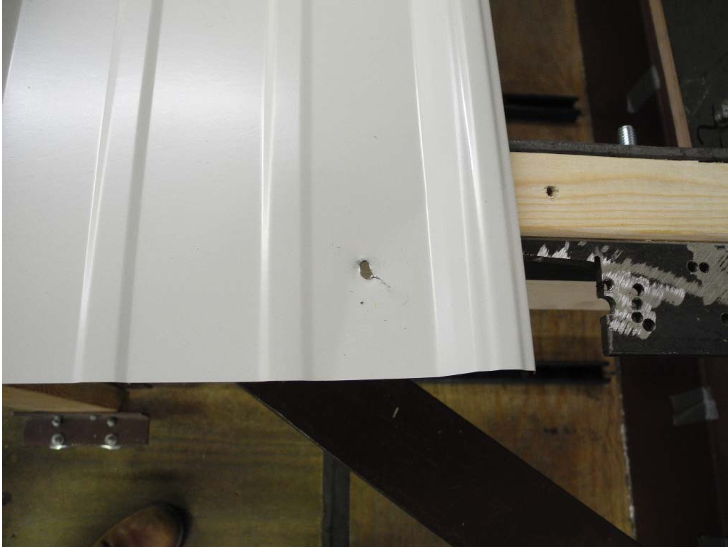
PHOTO 5 View of panel slotting at fastener near the pinned support in Test #1. (DSCN1017)
